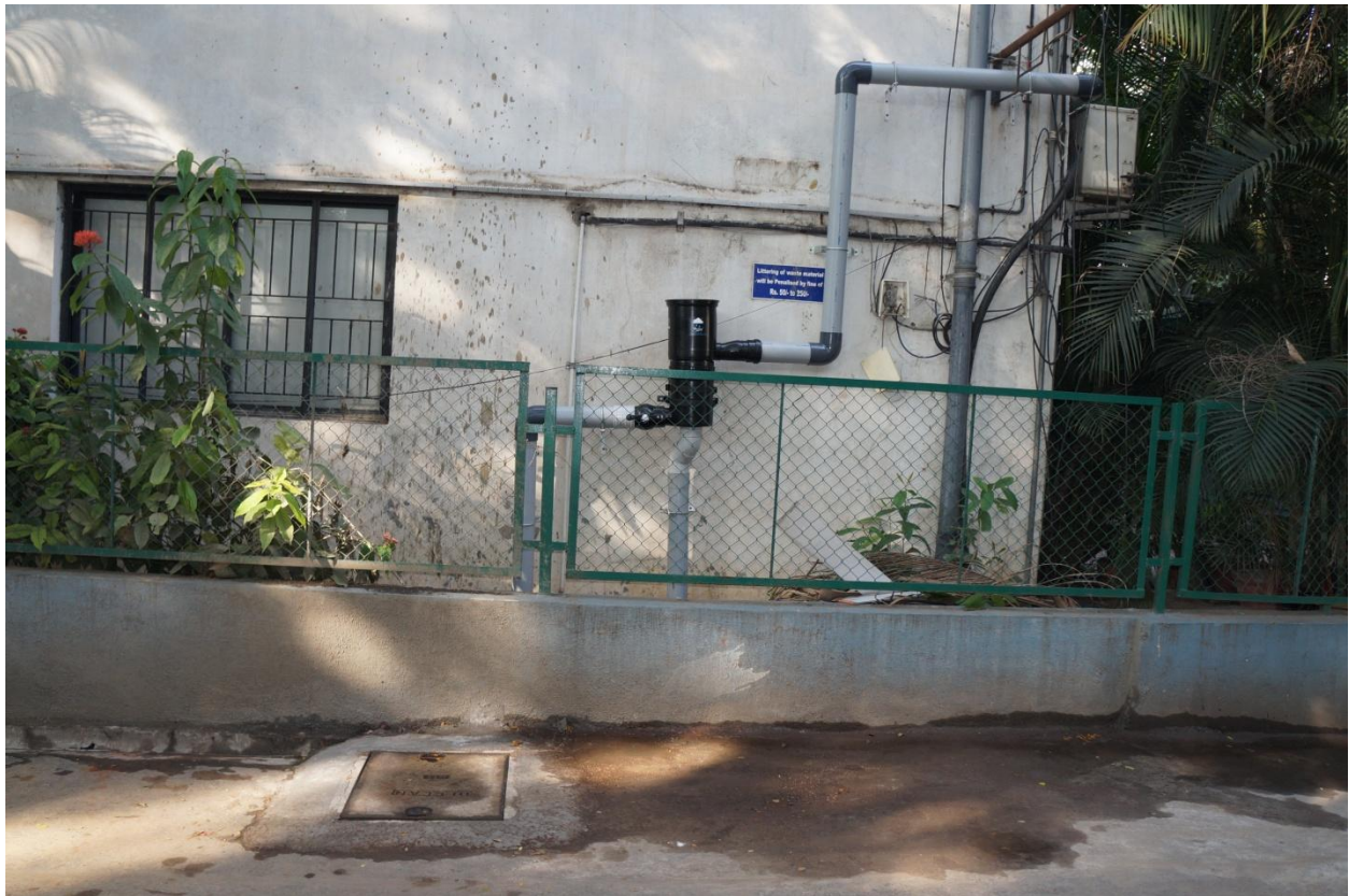
Rain water Harvesting utilisation in the campus
